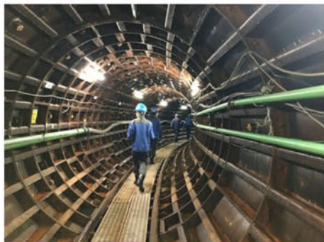
On-site inspection inside a tunnel where a water pipeline is being newly installed.
