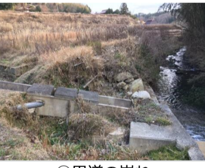
③②③里道の崩れ
