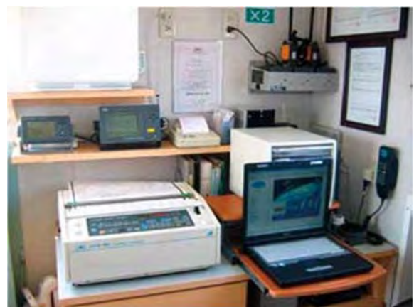
無線区画－2／Radio equipment area-2
