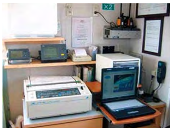
無線区画－2／ Radio equipment area-2
