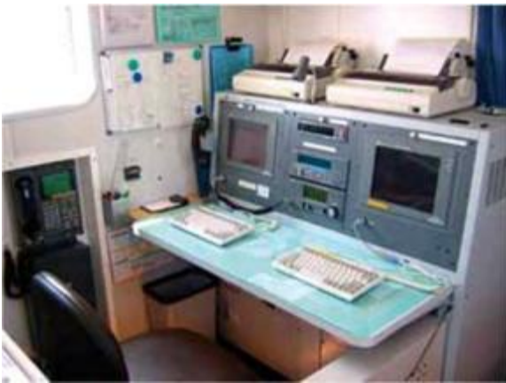
無線区画-1 / Radio equipment area-1
