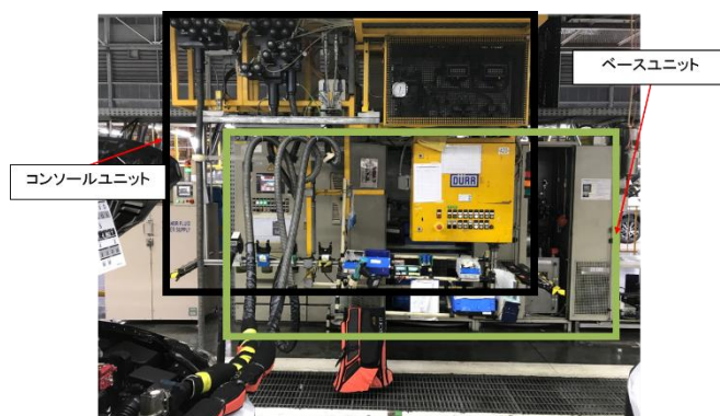
Fig.3 Radiator Fluid Filling Machine
